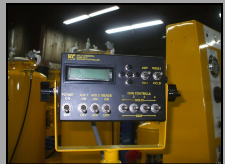
Serviced M40D Skipline Controller
