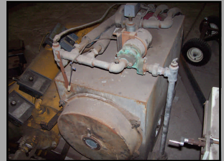
225,000 BTU diesel fired boiler with Wayne 12VDC burner.
