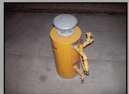
65,000 BTU propane fired boiler
